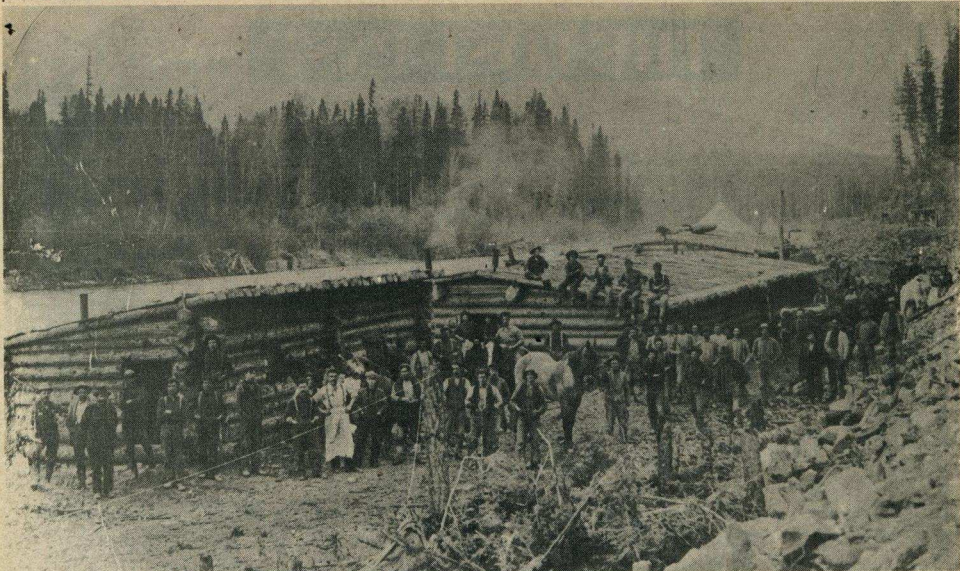
Typical construction camp during building of the Crow'snest Pass line. Workers testified that some of the bunkhouses were more like hospital wards. In some cases, men slept in tents, without stoves — in January
